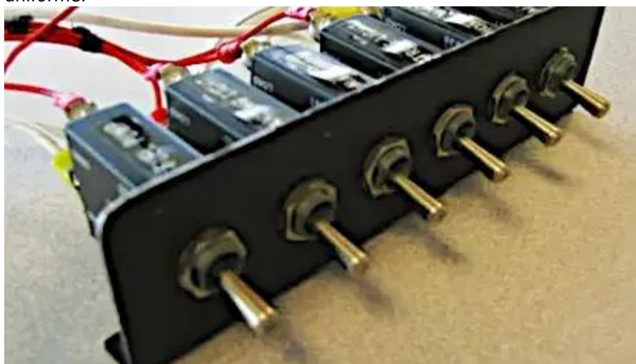
A view of the switch/circuit breakers from the front of the panel.
